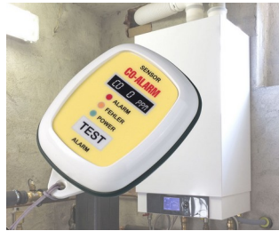
CO Gas Alarm
